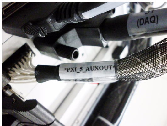
Figure 4-3 Interface cable label example (*PXI_5_AUXOUT*)
