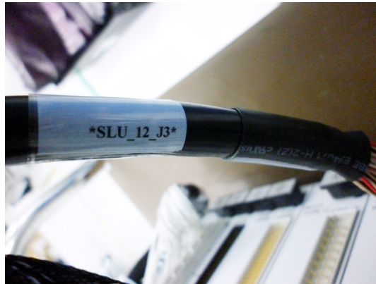
Figure 4-2 Interface cable label example (*SLU_12_J3*)
